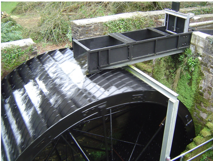
The former Brent Canvas Mill wheel in Devon, now used for domestic power generation.
